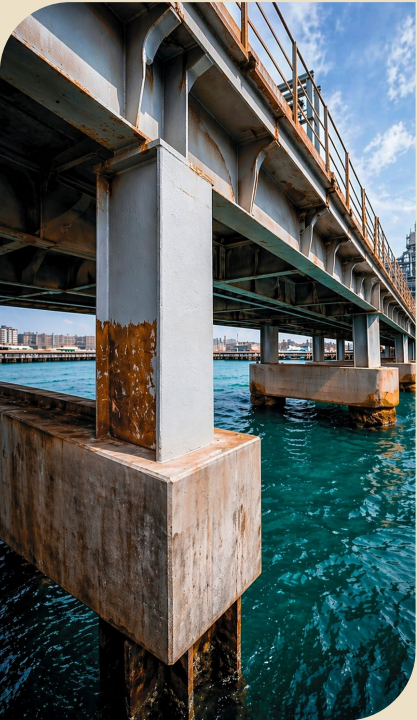
Corroding steel and concrete infrastructure in harsh environments requires advanced and sustainable protection solutions.
