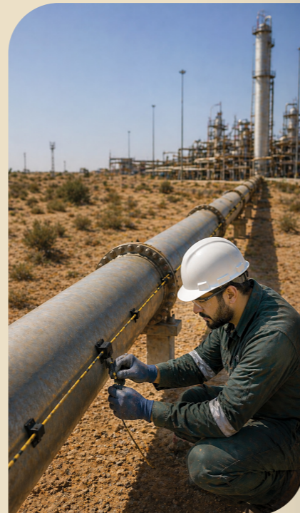
Distributed fiber-optic sensing system enabling real-time, AI-driven pipeline monitoring and anomaly detection.
