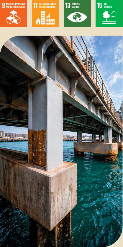
Corroding steel and concrete infrastructure in harsh environments requires advanced and sustainable protection solutions.
