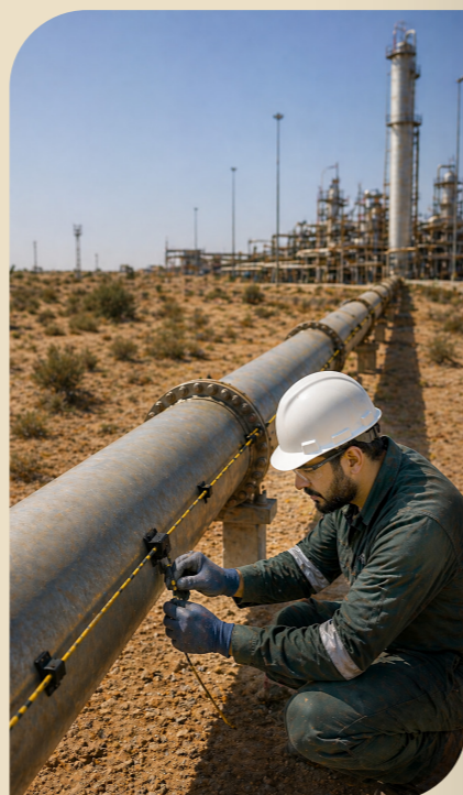
Distributed fiber-optic sensing system enabling real-time, AI-driven pipeline monitoring and anomaly detection.
